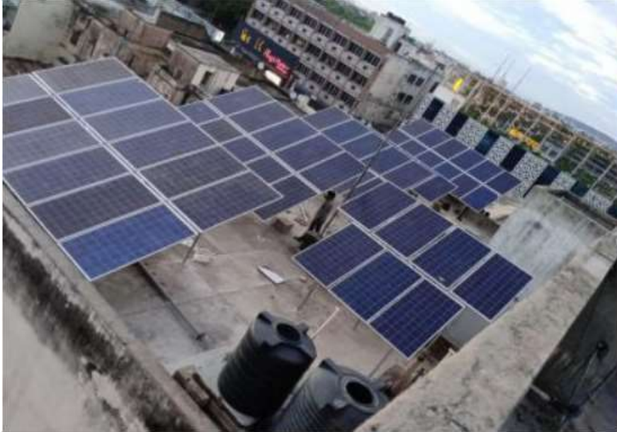
ICICI, MI Road, Jaipur Capacity – 20 KWp
