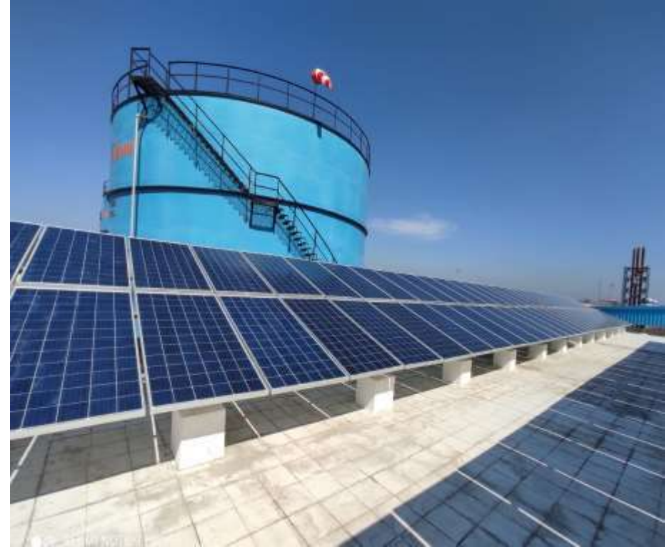
IOCL, Korba Capacity – 66 KWp
