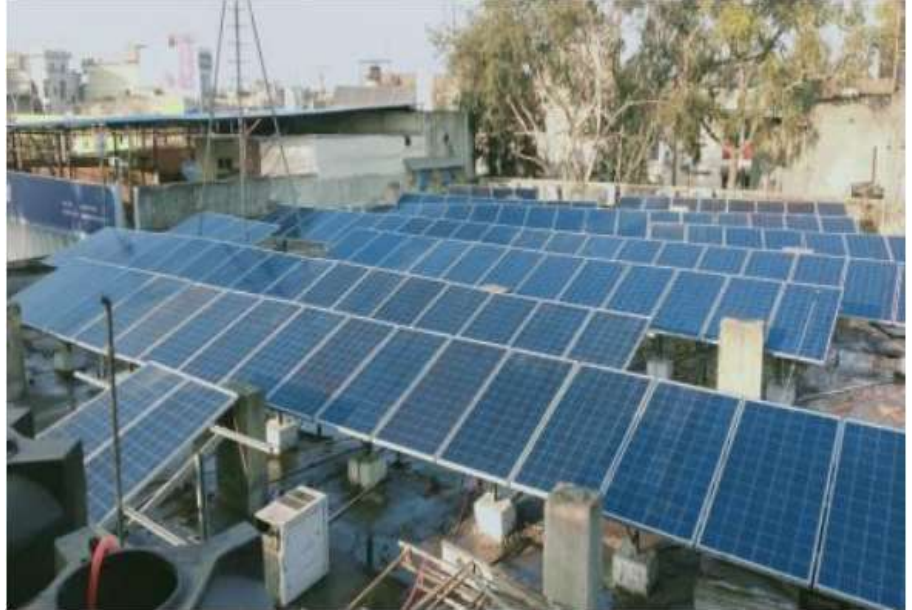
ICICI, Aerodrome Circle, Kota Capacity – 40 KWp
