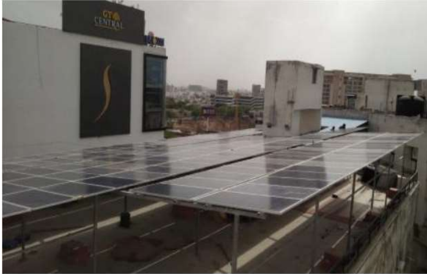
ICICI, JSEL, Jaipur Capacity – 55 KWp
