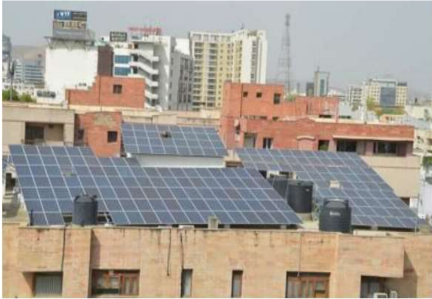
ICICI, SP Marg, Jaipur Capacity – 70 KWp
